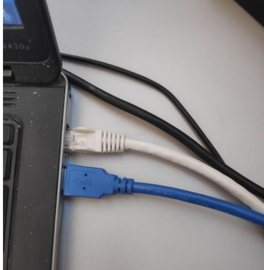
Figure 4-2: Laptop connections. The Ethernet cable comes from the switch. The USB3.0 comes from the PTZ camera
