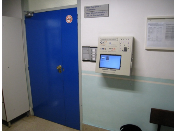
Fig. 4. Physical installation (at EUPMt) in a wall for door opening system.
